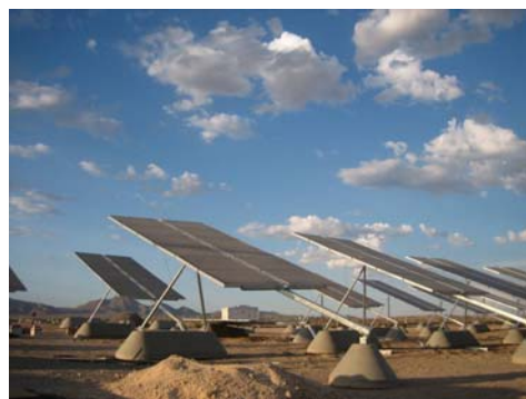
Figure 12: Nellis AFB 2.5MW Bifacial Tracker Installation
